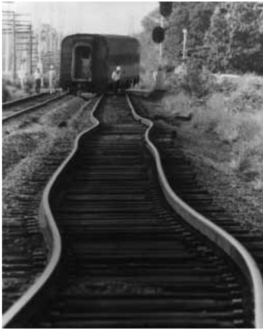
Thermal expansion: The extreme temperature of a July day in Asbury Park, NJ, caused these railroad tracks to buckle and derail the train in the distance. (AP/Wide World Photos)
