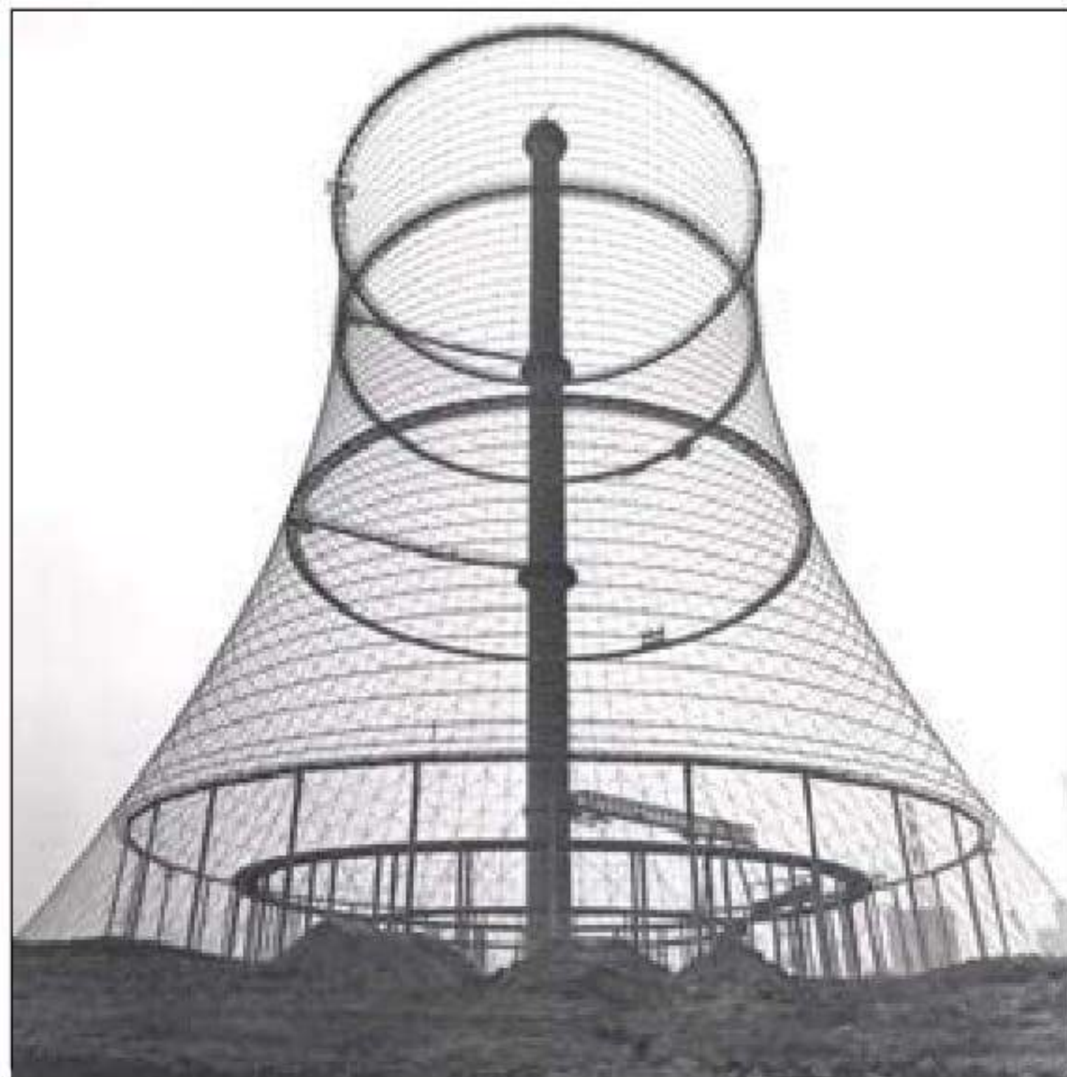
Fig. 2. Cooling tower Schmehausen [2], permanent
