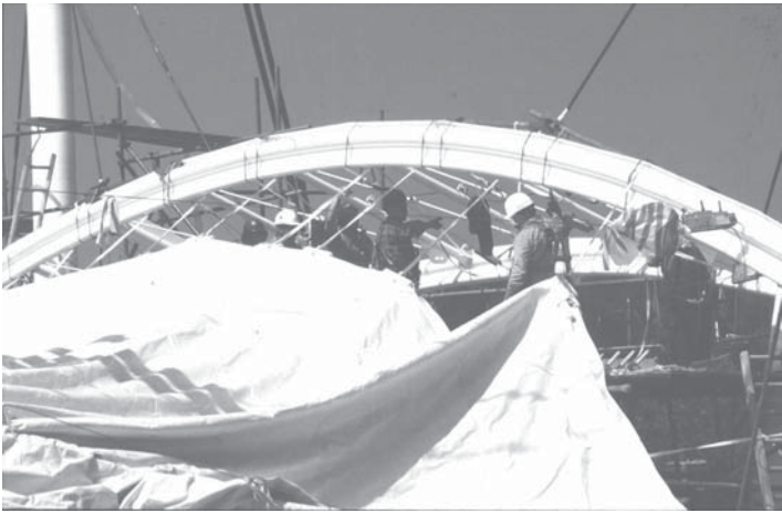
12.7 Stressing out the membrane at the Inland Revenue amenity building, Nottingham (photo: Alistair Gardner).
