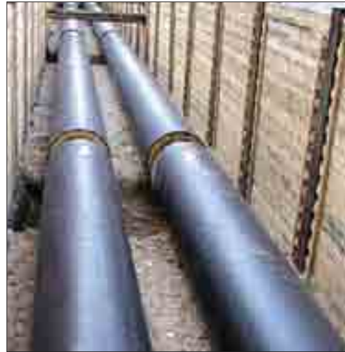
Cast iron pipes.
