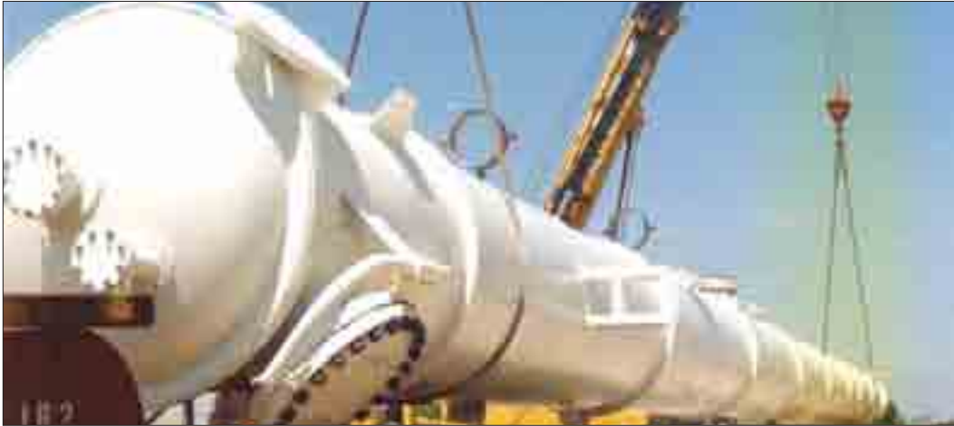
A long oil tank.
