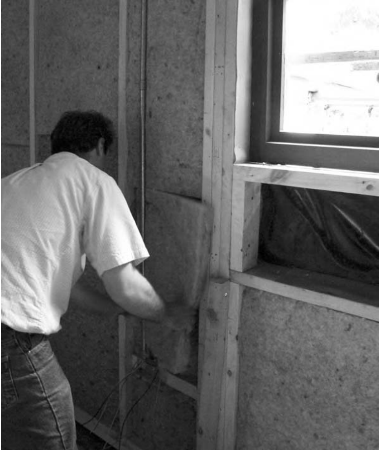
10.11 Wool insulation being installed in the wall of a new building. [Source: Second Nature Ltd, UK ]
