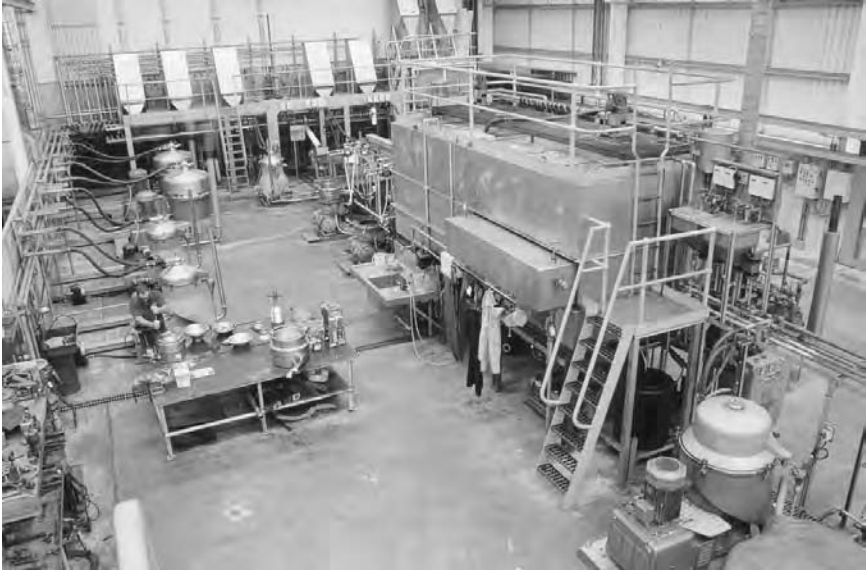
2.14 Woolgrease recovery plant. [Courtesy of Jandakot Wool Washing Pty Ltd.]
