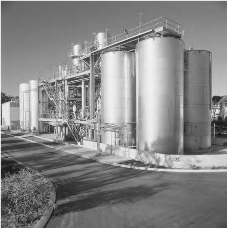
2.15 Effluent treatment plant incorporating an evaporation system. [Courtesy of Jandakot Wool Washing Pty Ltd.]
