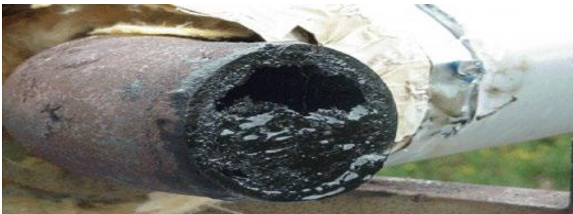
Figure 8.11 Pipe plugged with decomposed heat transfer fluid.
