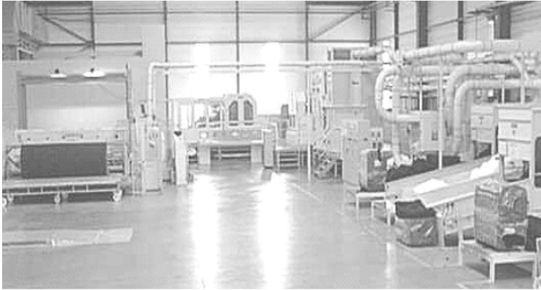
5.4 Mécaplast media manufacturing line.
